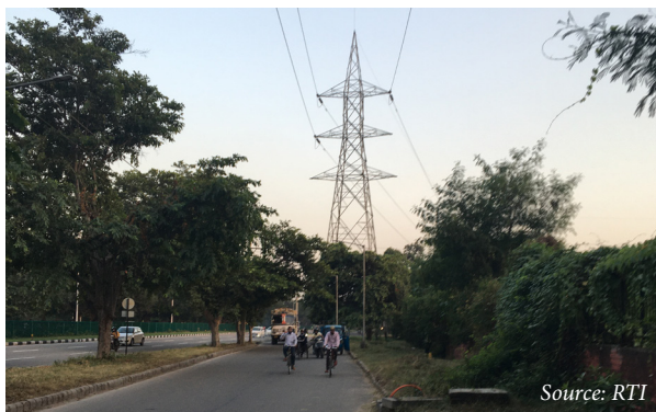
a) HT lines in Industrial Phase II, Chandigarh
