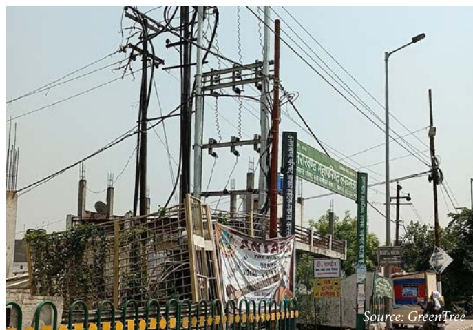
Figure 6.20: Status of Electrical Infrastructure in Lucknow
