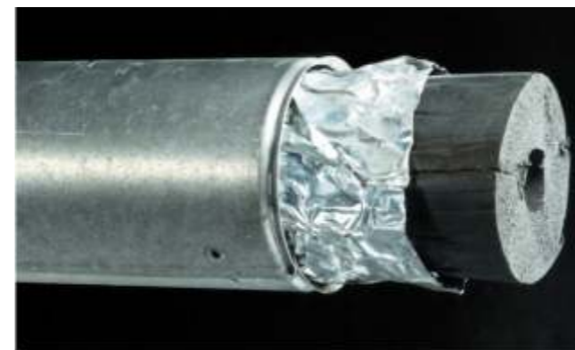
Fig14: Insulation of hot water piping
